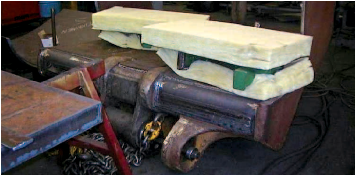
It may be justified to use mineral wool to slow down cooling in case of critical welding, see photo.
